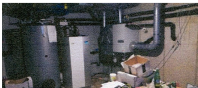
Fig. 2. Technical room of the building with the heat pump, storage tank and the mechanical ventilation system
